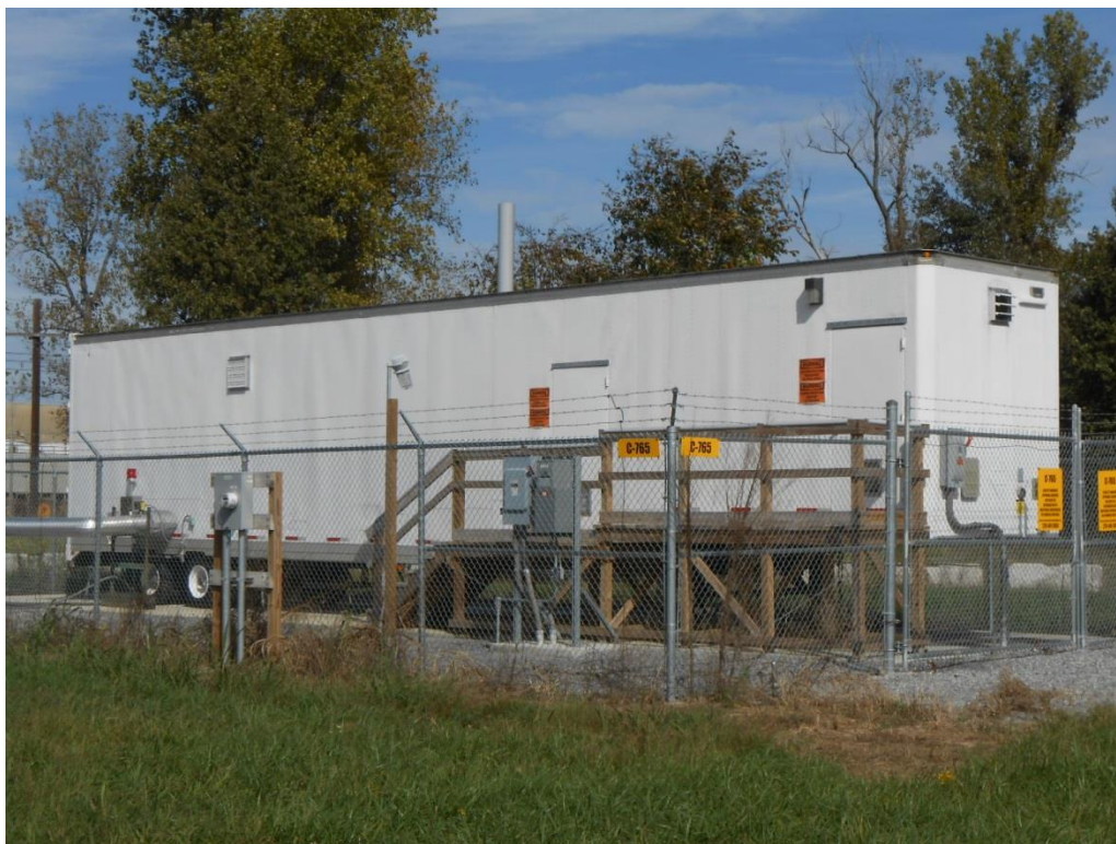
Figure 11. Northeast Plume Groundwater Treatment Trailer
